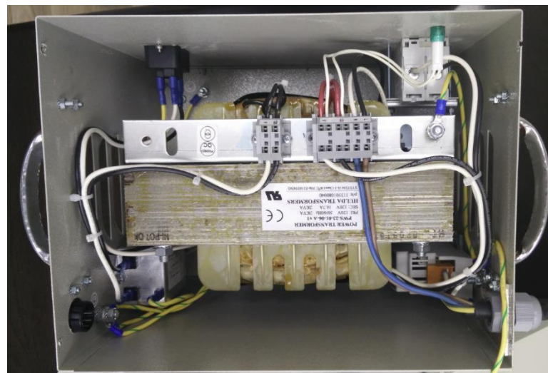
Fig.4 Isolation transformer box internal View
