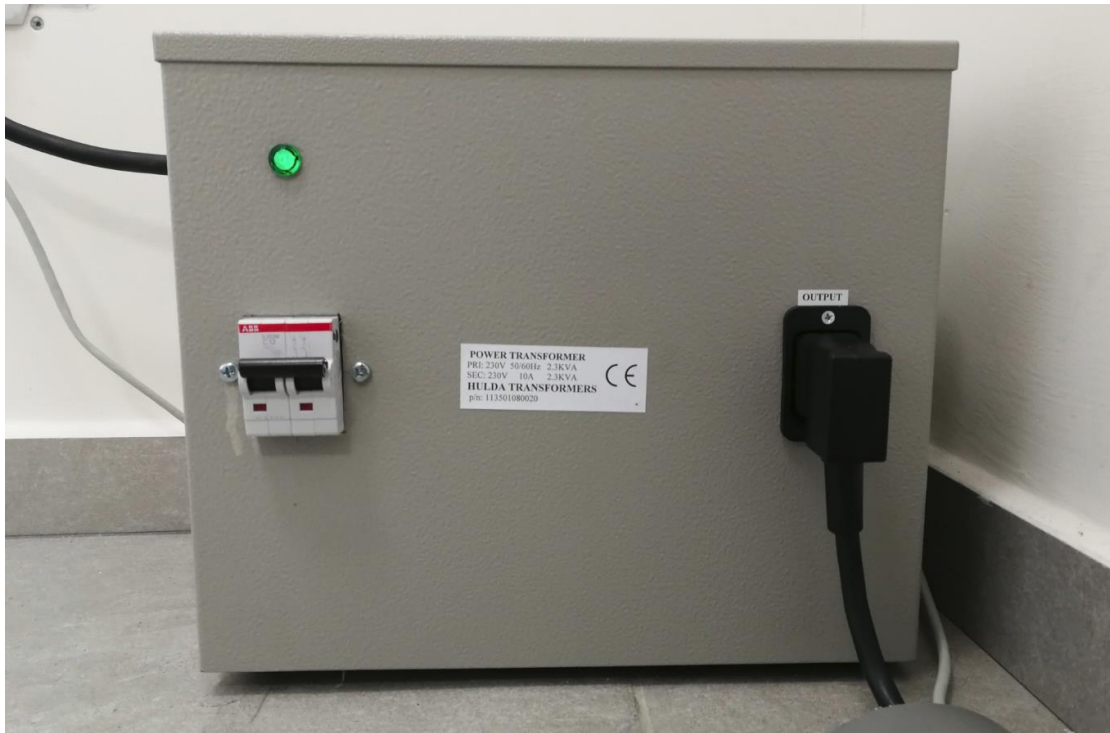
Fig.5 Isolation transformer box front View
